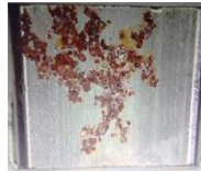
Figure 33. Rust on the surface of inductors.
